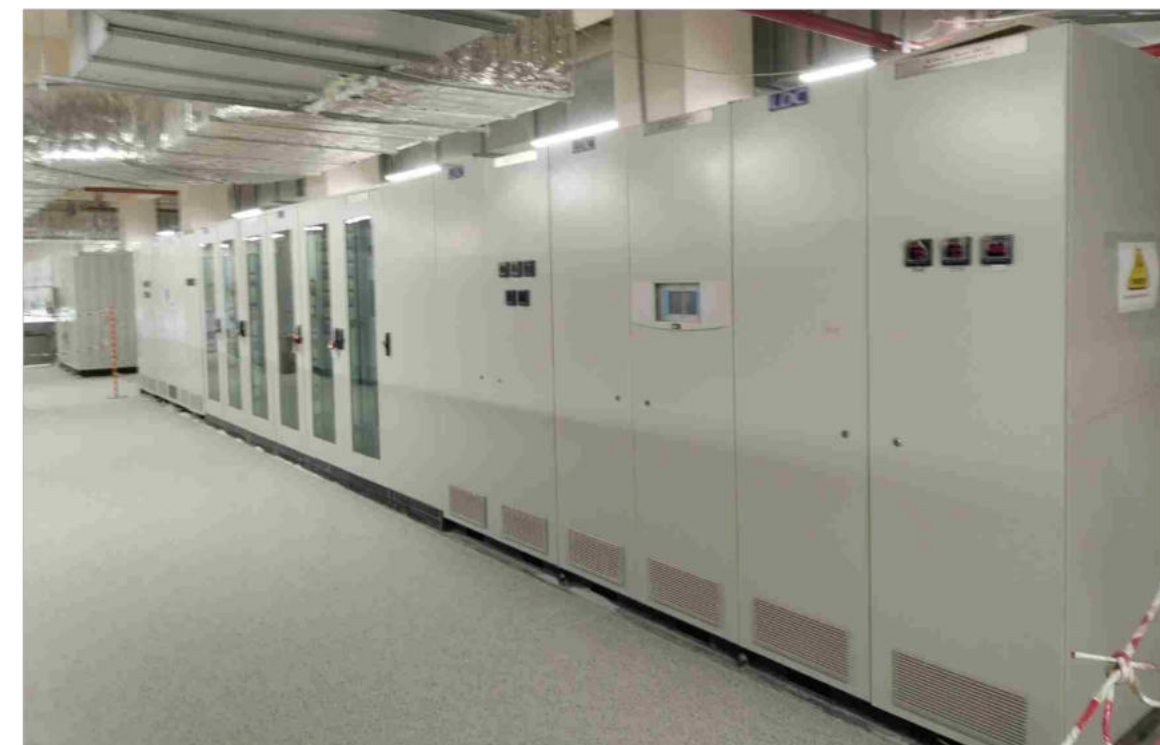
Uzbekistan Syrdarya 1500MW Gas Combined Cycle Independent Power Plant Project - Site Photos
